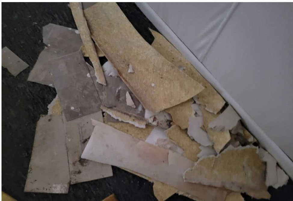
Photo 8: View of positive vinyl sheet flooring debris pile in building 211 1 st floor west side office located in middle room and under carpet and shower.
